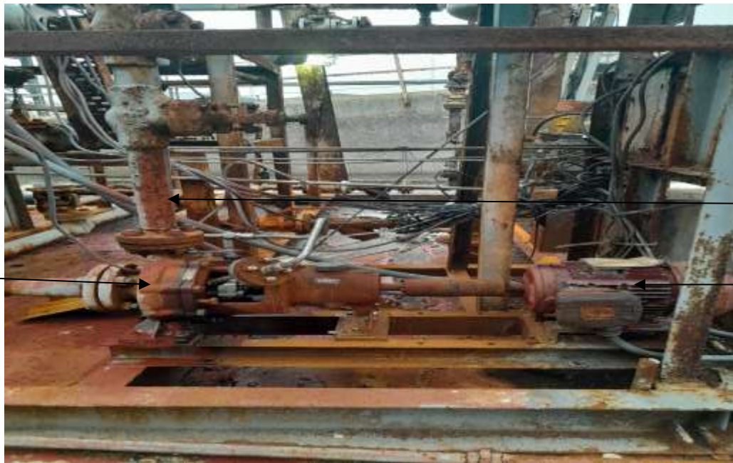
Figure 3: shows the model pump before installation of pressure controller, pressure transmitter and solenoid valves
