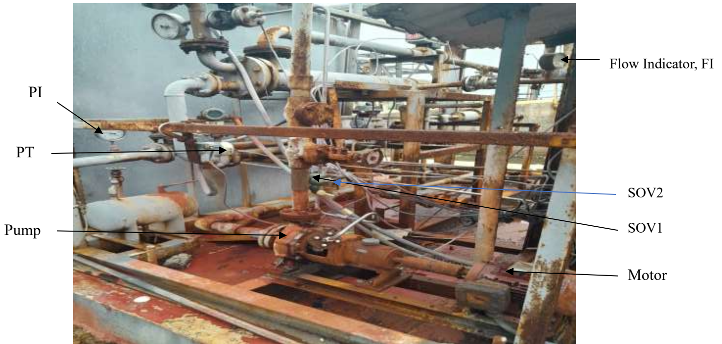
Figure 4: The model pump after installation of pressure controller, pressure transmitter and solenoid valves
